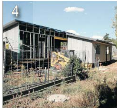
ALMOST THERE: The second piece of the house sits ready to be assembled on Tuesday.
