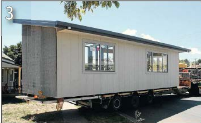
PAITIENCE: The first part of a house for Pat and Helen McDermott is carefully guided into place on Tuesday afternoon. Pictures: Declan Rurenga
