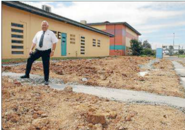
ROOM TO MOVE: GEO Group general manager Andy Walker inspects the foundations for the new women's remand building under construction at the Junee Correctional Centre.
